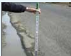
Road edge defect – condition deficiency
