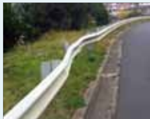
Road guard rail – maintenance required?
