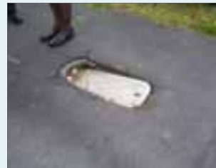
Utility pit on Council asset – safety issue
