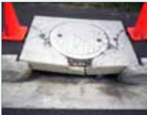
Water pipe cracked – serviceability issue and road damage
