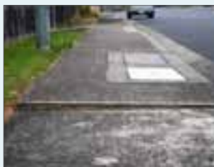
Footpath trip – >35mm step – safety deficiency
