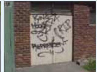
Graffiti – aesthetic and cleanliness deficiency
