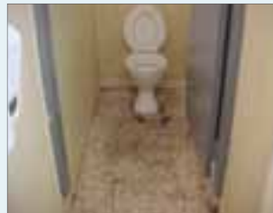
Toilet facility – aesthetic and cleanliness deficiency
