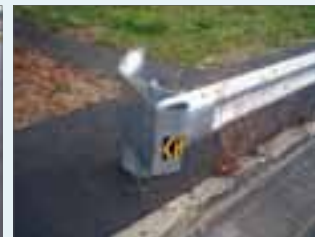
Road guard rail – maintenance required?
