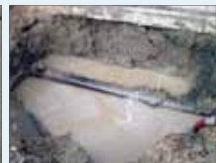
Water pipe cracked – serviceability issue and road damage
