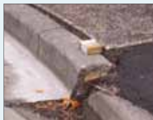
Disjuncted curb – >40mm – functional deficiency
